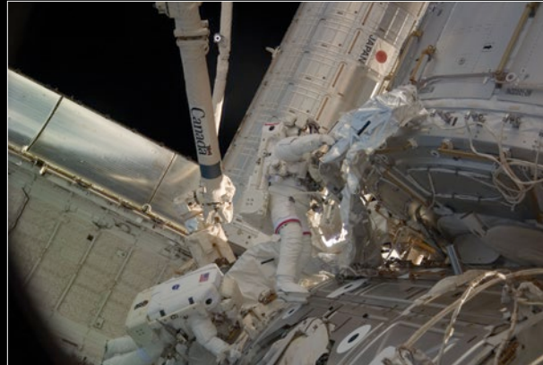
Figure 14. Bob Behnken and Nick Patrick installing ammonia lines and associated insulating blanket during the second STS-130 spacewalk. Limited consumables dictated that the installation plan proceed precisely according to schedule to ensure enough clean-up time after the predicted ammonia leakage time frame.
