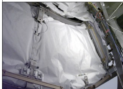
Once all the equipment that needs to be attached to the pressure shell or run under the insulation blankets is installed, the blankets themselves are installed. These blankets are a thick composition made of materials such as Nextel® and Kevlar®. These materials not only insulate the pressure shell, they serve as another debris barrier where MMOD energy is dissipated and debris is broken into smaller fragments. This photo shows some of the MLI blankets on the Joint Airlock.
