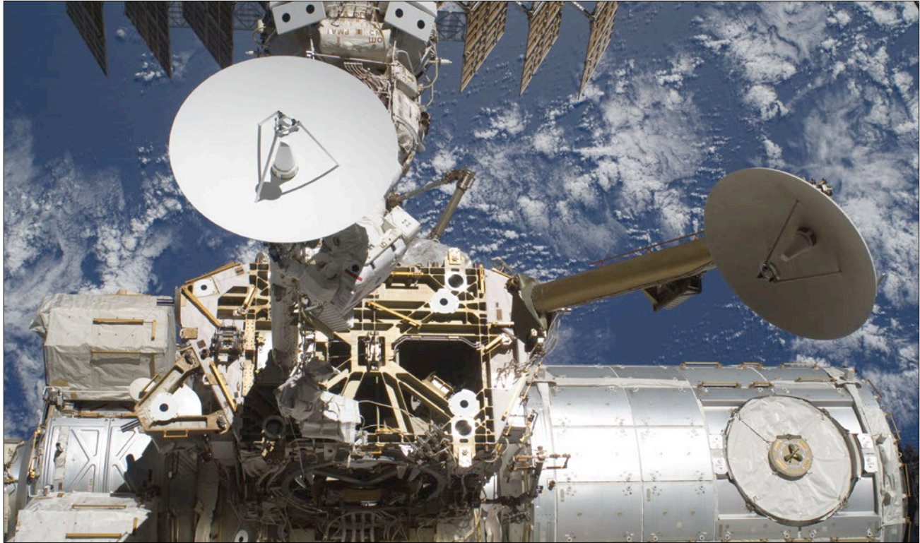
Figure 3. STS-132/ISS-ULF4 mission specialist Steve Bowen works to install the backup Space-to-Ground Antenna (the white radio dish near the top left of the figure) on the Z1 truss (located next to the original antenna, which is angled to the right).
