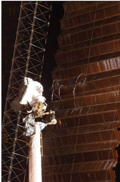
Figure 22. Parazynski, partway through the repair. Three of the five required cufflinks are installed.
